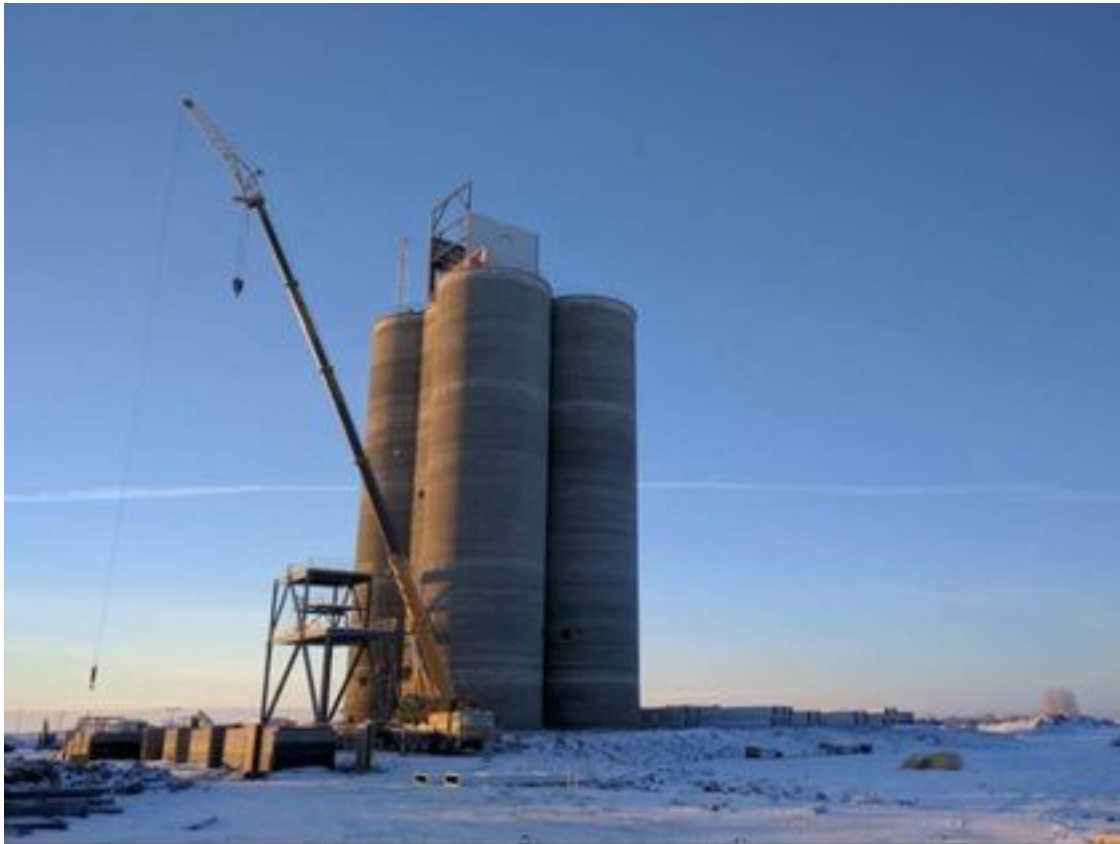
GrainsConnect Canada's high-throughput grain terminal under construction in Maymont, Sask., 90 kilometres northwest of Saskatoon. SUPPLIED
